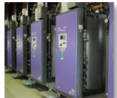
LNG boilers began operation in Komaki Plant
