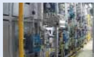
Regenerative burners installed in the upper and lower faces of the kilns
