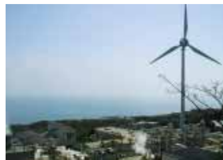
The Tokyo Electric Power Company (TEPCO) has been entrusted by the New Energy and Industrial Technology Development Organization (NEDO) since March 2001 to conduct testing of NAS® batteries on the island of Hachijojima in conjunction with wind power generation facilities.
