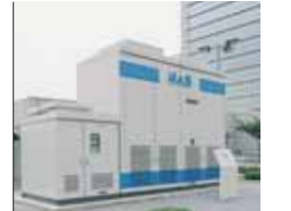
NAS ™ battery energy storage system (Nagoya Plant)
