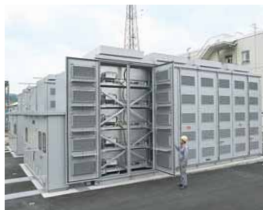
NAS™ battery (sodium sulfur battery) energy storage system
