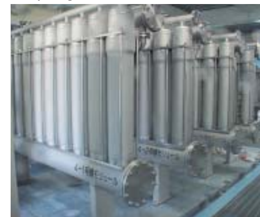
Large ceramic membrane water purification system
