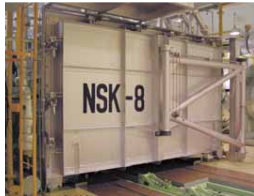
NSK-8: Regenerative burners boost combustion efficiency by storing heat (Nagoya Plant)
