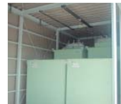
Storage vault for equipment containing PCBs (Chita Plant)
