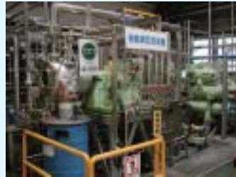
Copper sulfate recovery equipment (Chita Plant)
