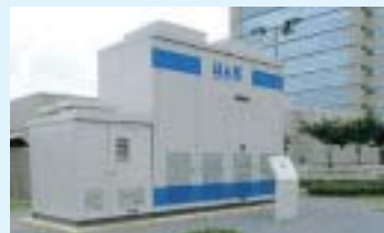
NAS ® battery (Nagoya Plant)
