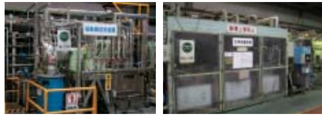
Copper sulfate recovery equipment
