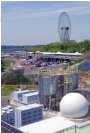
NAS® batteries at the New Energy Plant (below left) and the Methane Fermentation System
