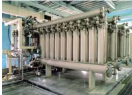
The first large-scale ceramic membrane water purification system ordered, by the Tokyo Bureau of Waterworks in July 2001
