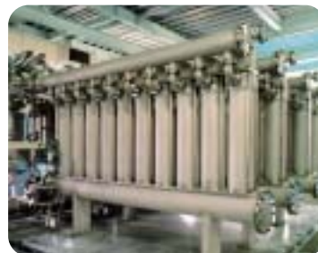
A ceramic membrane water purification system
