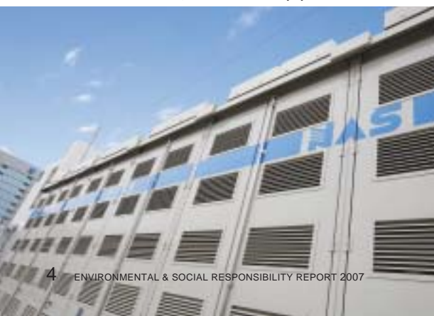
A 1,500 kW NAS ® battery system at the NGK AC Plant
