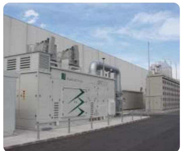
System combining fuel cells (front) and NAS® batteries (rear)
