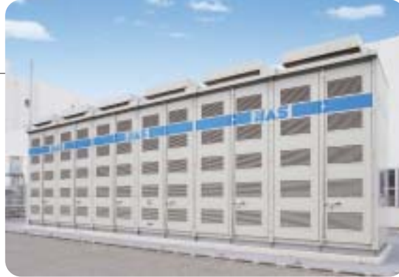
NAS® batteries for power storage
