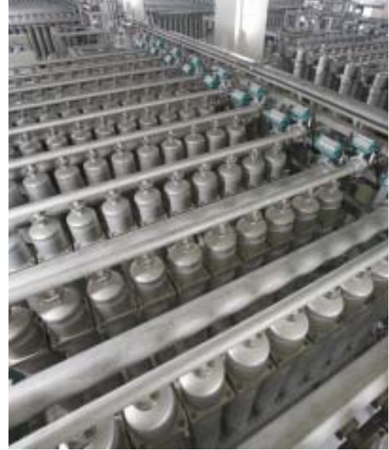
The water purification facility utilizes 1,800 ceramic membrane elements
