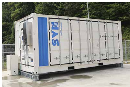
ENA ELECTRIC POWER, Yoshida Power Plant
